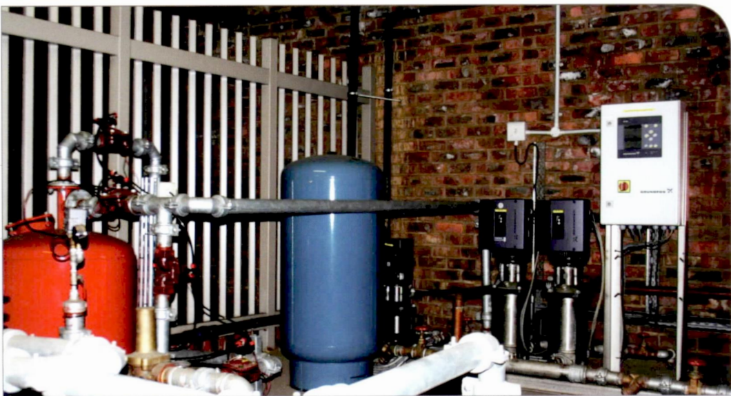
The rainwater harvesting system and pumps.
